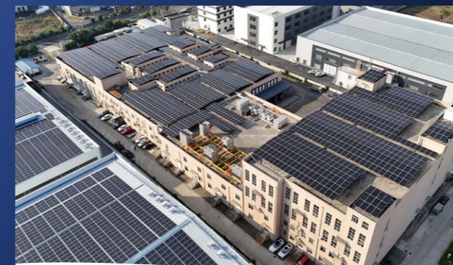
Industrial Park, Myanmar 1.24 MW PV + 1.5 MWh BESS
