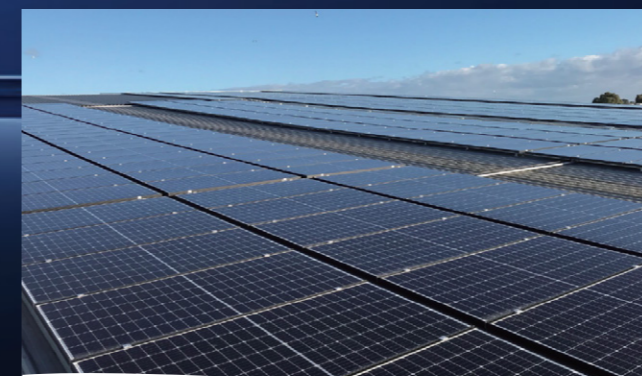
Farm, Panama 700 kW PV + 1.2 MWh BESS
